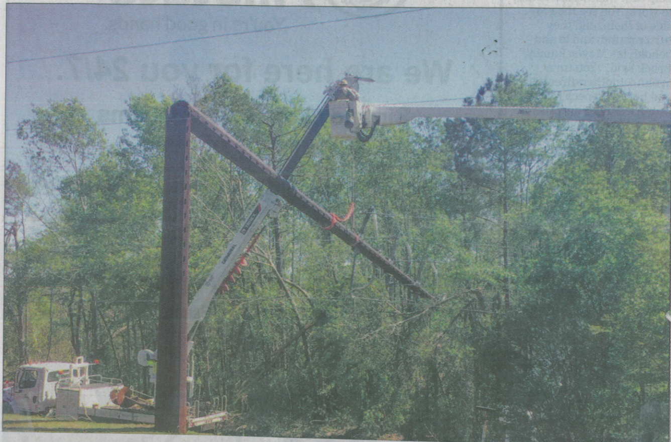
Workers spent Tuesday replacing four steel poles on a South Radio Station Road transmission line damaged by Monday's tornado that struck the Seneca area and left a number of residents without power. GREG OLIVER | THE JOURNAL
