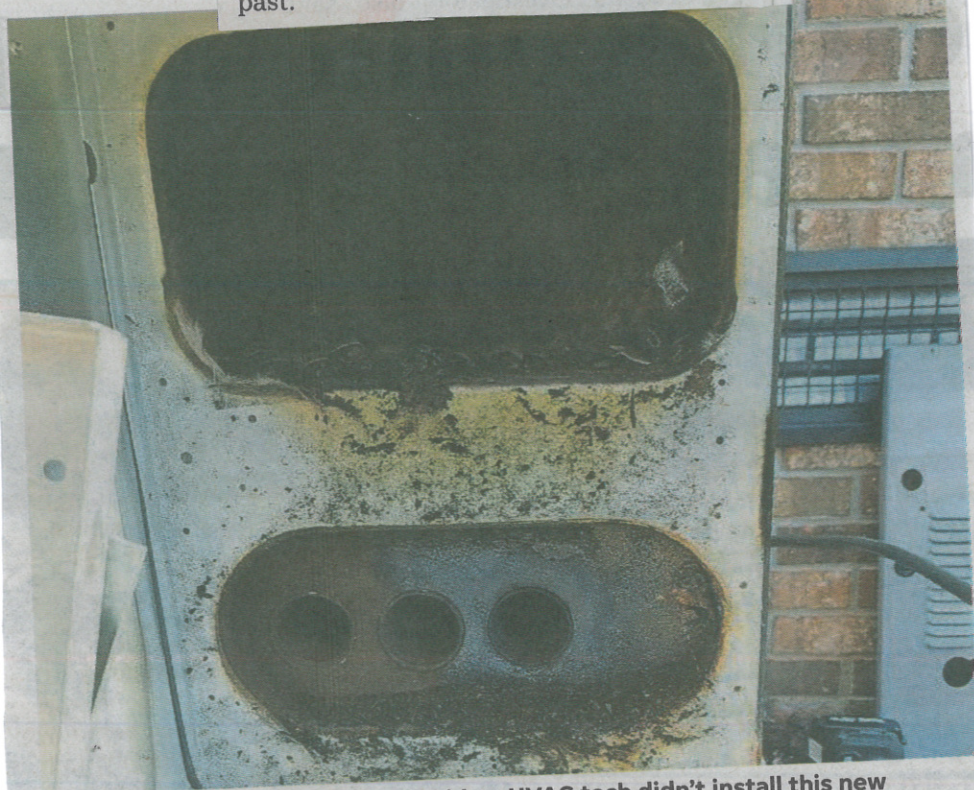
Jonathan Clark of Travelers Rest said an HVAC tech didn't install this new propane heating system properly, which led to more repairs and a carbon monoxide leak in his home. COURTESY OF JONATHAN CLARK
