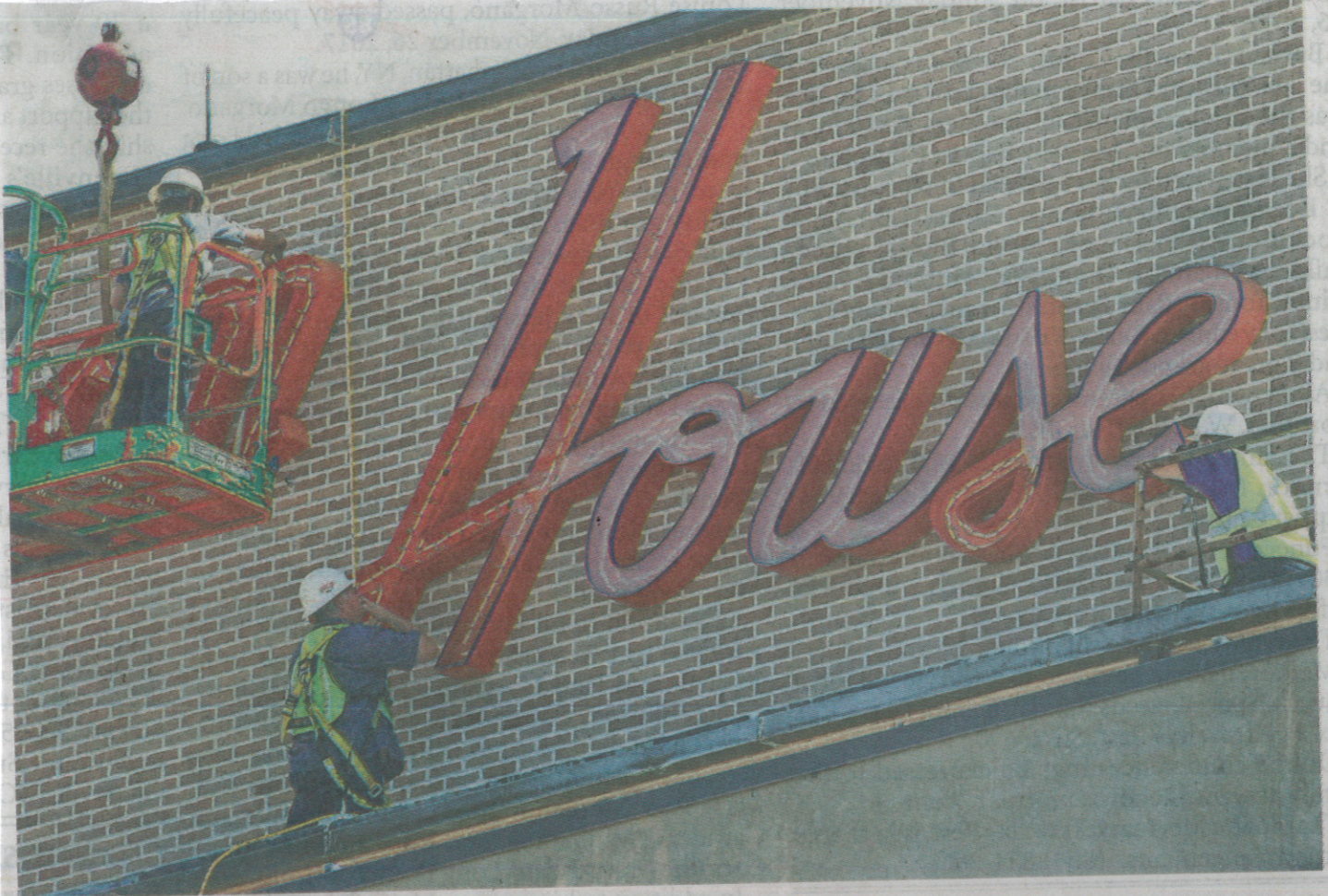
Workers remove the Clemson House sign in July. The house will be imploded this weekend. KEN RUIINARD/INDEPENDENT MAIL
