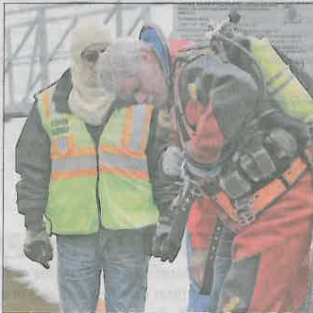
A commercial diver emerges from the Seneca River at Martins Creek Landing after attaching cables to a submerged Lincoln Navigator that rolled into the river Wednesday morning.
