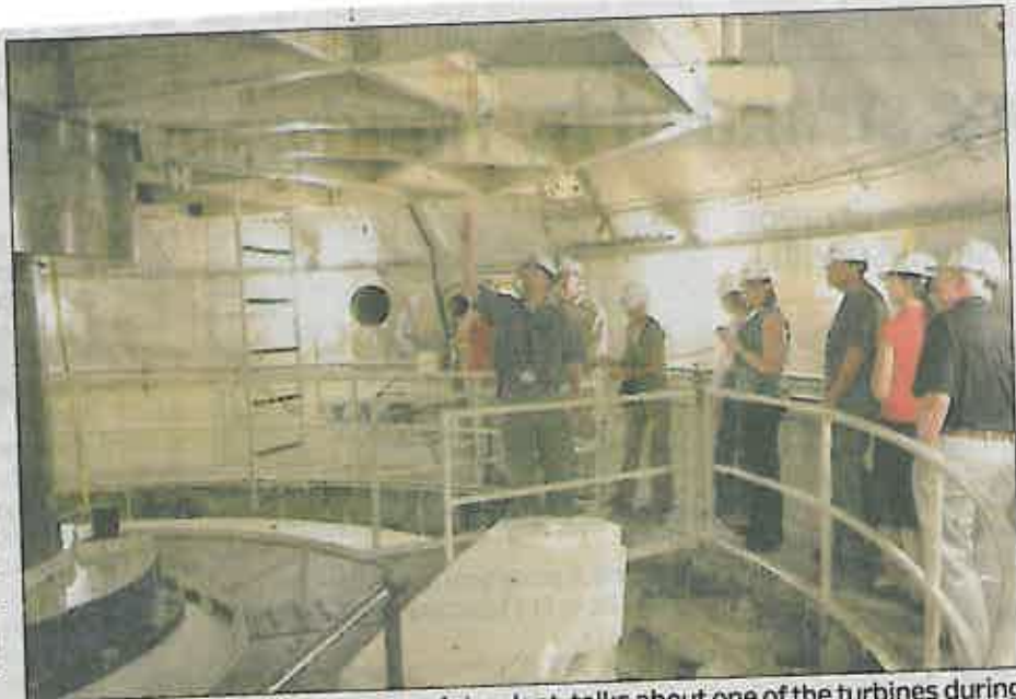
Chad Luce, Jocassee Station superintendent, talks about one of the turbines during a tour of the Jocassee hydro station with federal energy officials and others involved in relicensing of Duke's hydro projects on Jocassee and Keowee.
