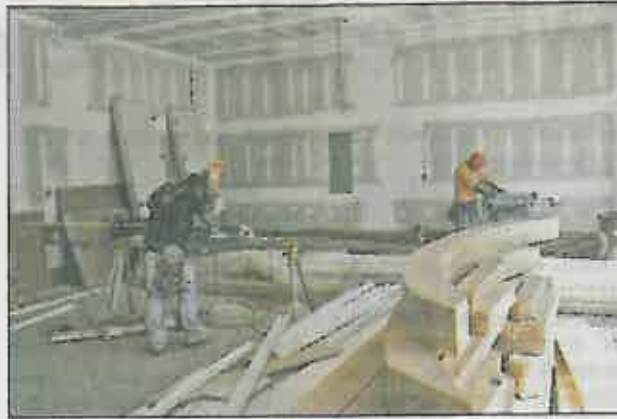
Construction workers build a home in Claremont, a subdivision off Roper Mountain Road. KEN OSBURN/STAFF
