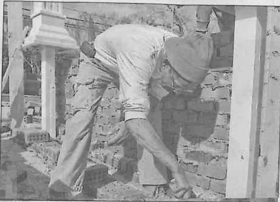
Brick mason John Williams performs work on a sign base on Washington Street in Greenville. PATRICK COLLARD/STAFF
